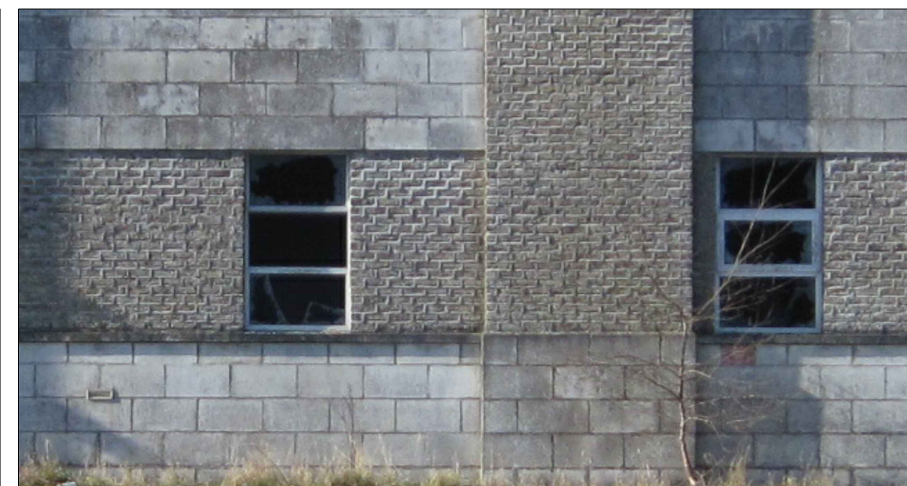
BRICK & STONE DETAILS - OFFICERS MESS BUILDING STONE PLINTH AND HEAD DETAIL WITH BRICK-FILL/SPANDREL BETWEEN WINDOWS
