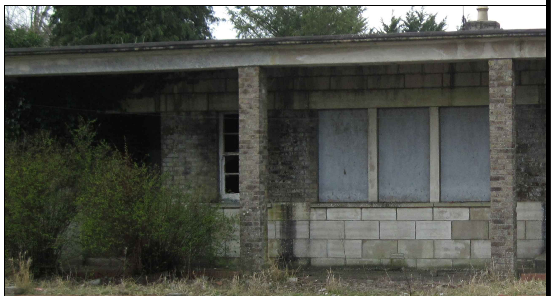
BRICK & STONE DETAILS - SMALLER BARRACKS BUILDINGS STONE PLINTH AND HEAD DETAIL WITH BRICK-FILL BETWEEN WINDOWS
